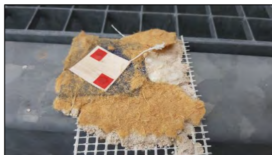
Figure 45 : Removed render layer of variant N 2.6 (dark render) with Balsa sensor and wood fibre residues: No fungal mycelium visible.
