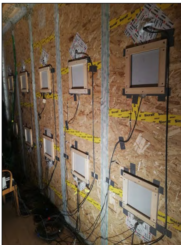
Figure 20 : Measurement setup of a heat flow measurement with heat flow meters and surface temperatures (constellation 1).
