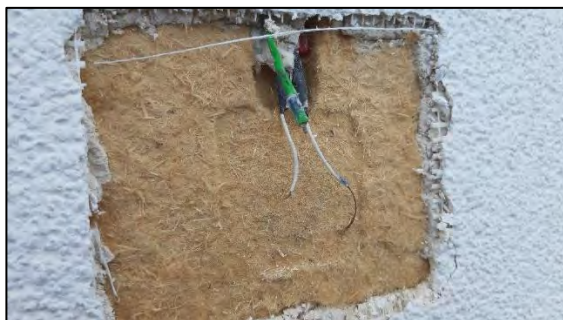
Figure 42 : Opened measuring position P at variant N 2.3 (bright-coloured render) after the test period. No fungal mycelium visible.
