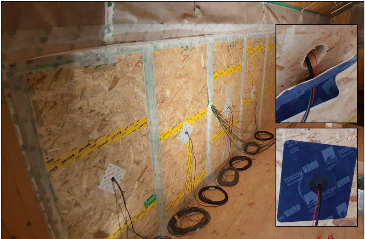
Figure 16 : Frontal installation of the combination sensors (measuring position "a").
